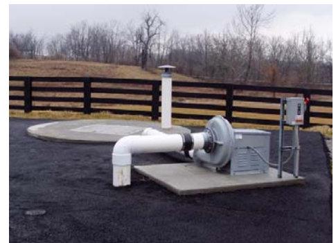
Underground Odor Control Unit
