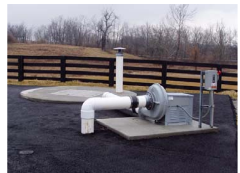
Underground Odor Control Unit
